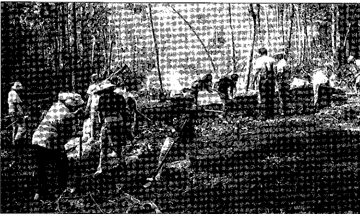
18 volunteers from Trinity Baptist Church, Harriman, Tn., dug the footers and poured the concrete for the new house.
