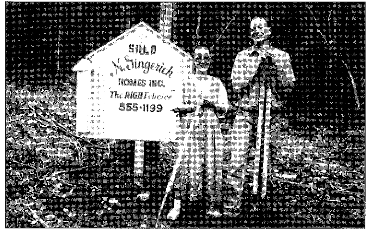
Mike & Lori McFerren, Wichita, Ks., put in plumbing and the walls for the office bathroom. Lori makes great "fruit shakes!"
